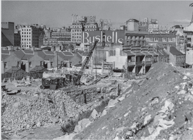
FIGURE 6 Excavation through The Rocks for construction of the Cahill Expressway's southern approach to the Sydney Harbour Bridge in 1955.
