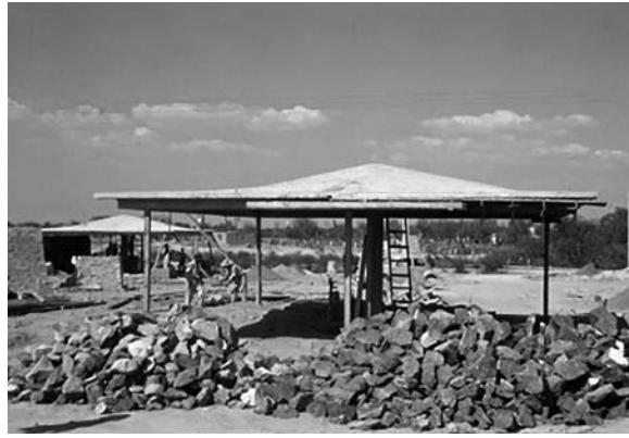
Félix Candela, casa económica tipo, en construcción, Monterrey, Mexico, 1959. Foto: Department of Rare Books and Special Collections, Princeton Library.
