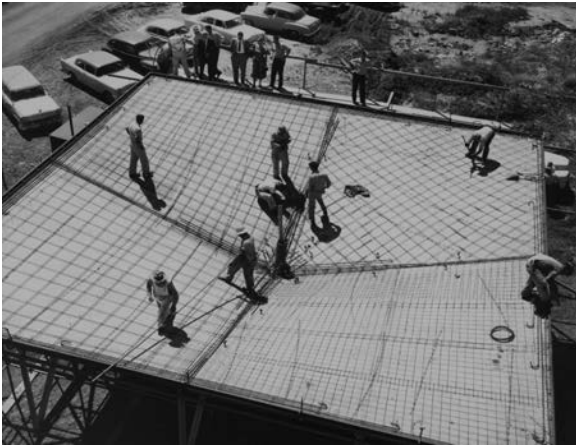
Montando la prueba del primer paraguas americano, en Colorado, 1956. Foto: Félix Candela Architectural Records and Papers, Dept. of Drawings & Archives, Avery Architectural and Fine Arts Library, Columbia University.
