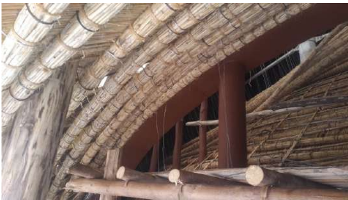
Fig. 26. Careful integration of materials and techniques in reconstructing the Main House or Muzibu Azaala Mpanga, Kasubi Tombs complex, Kampala, Uganda (Source: Jonathan Nsbuga)
